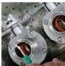
Service tank valves
